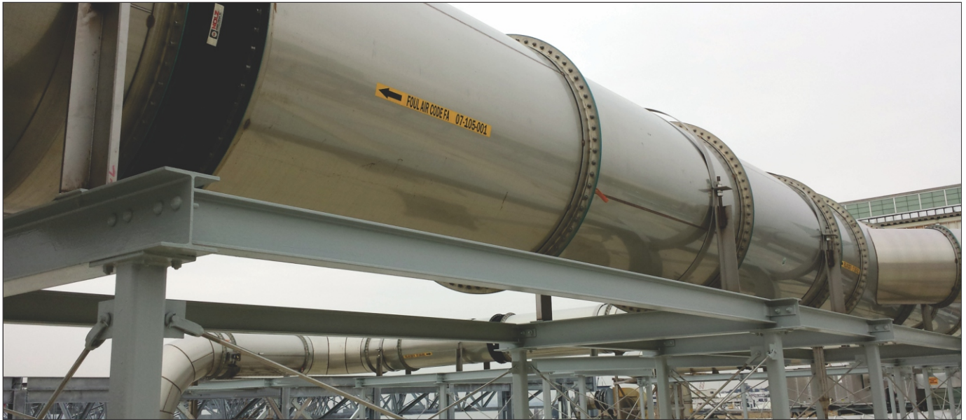
PSP® odor control duct rooftop installation at District of Columbia Water and Sewer Authority
