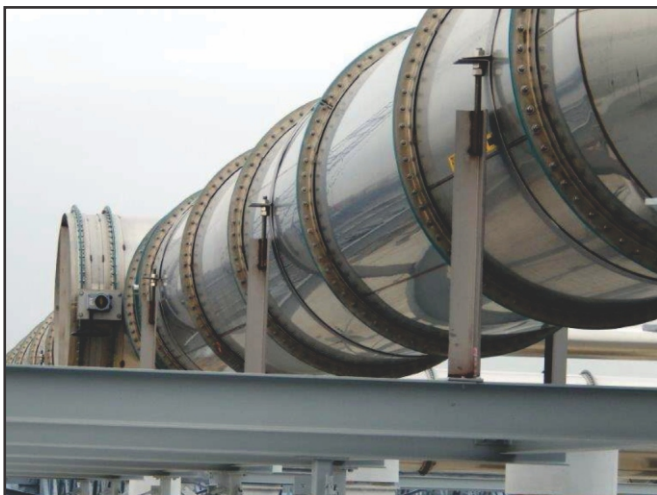
Another view of Blue Plains dewatering facility odor control duct.
